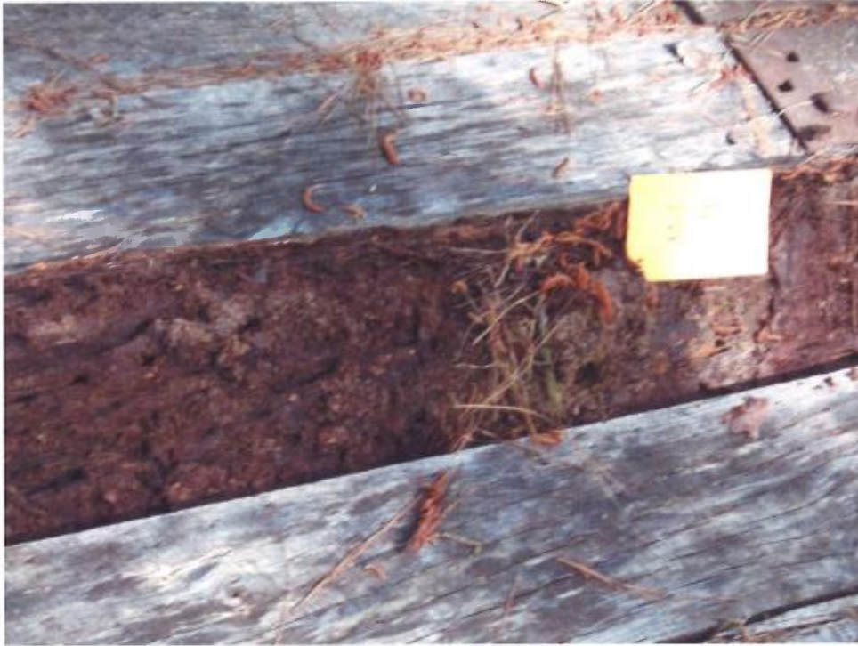
Figure 2 - Tie #25 with decay and beetle damage.
