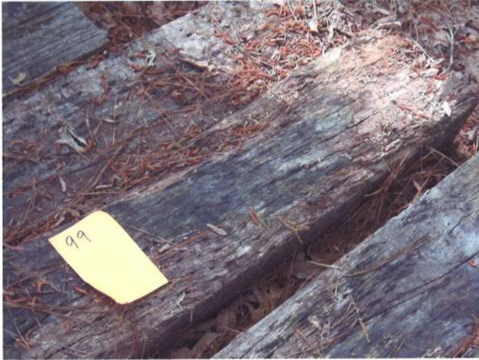
Figure 4 - Tie #99 with decay on upper surface.
