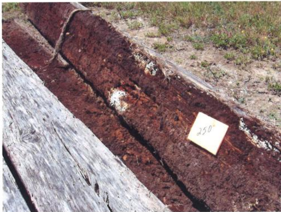
Figure 9 - Tie #250 with heavy decay and trace termite damage.
