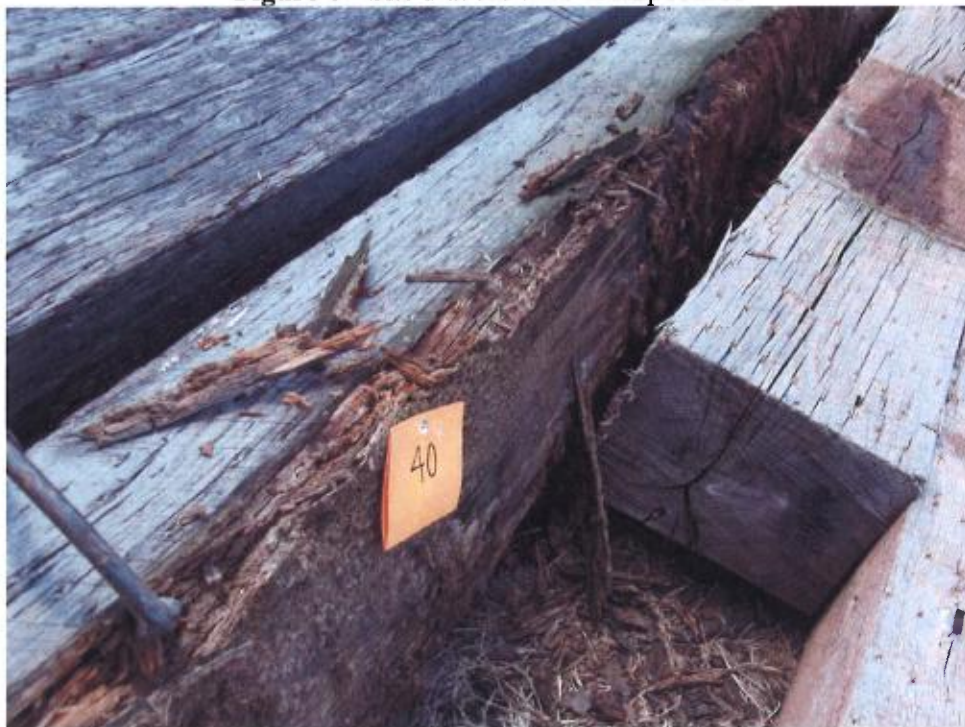
Figure 7 - Tie #40 with decay.
