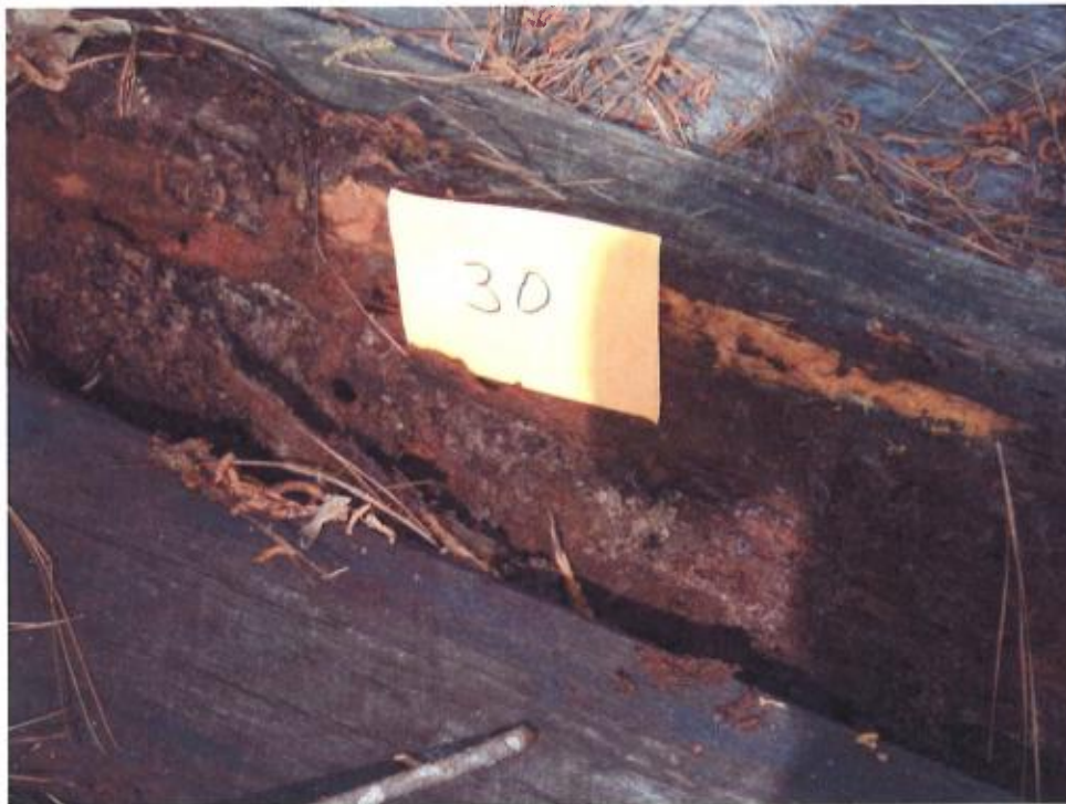
Figure 3 - Tie #30 with decay damage.
