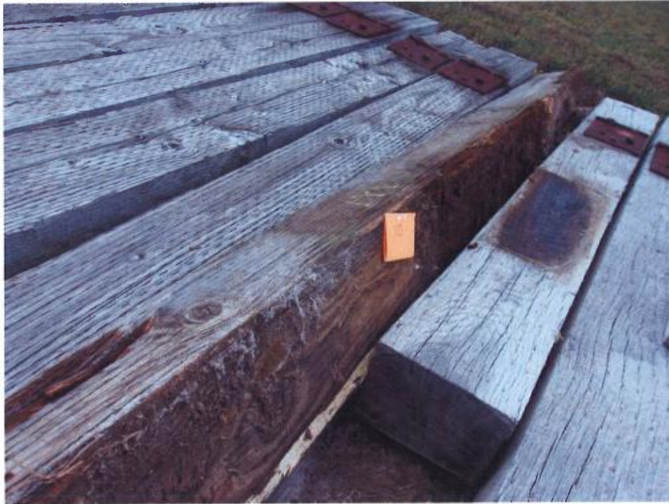
Figure 8 - Tie #110 with decay and trace termite attack.
