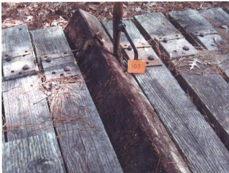
Figure 5 - Tie #103 with moderate decay.
